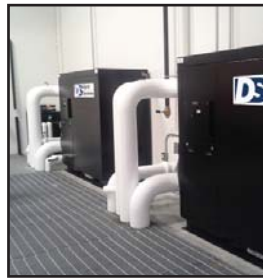
Coolant Storage and Distribution
