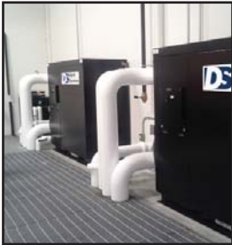
Coolant Storage and Distribution
