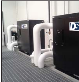
Coolant Storage and Distribution
