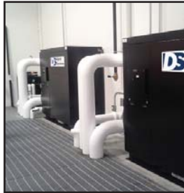
Coolant Storage and Distribution
